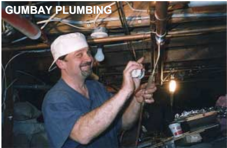
Vince Paruta volunteers to fix a leaky pipe in our lodge in Vermont.
